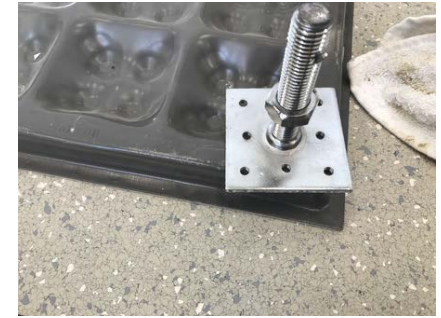
Raised Access Floor issues remain outstanding
